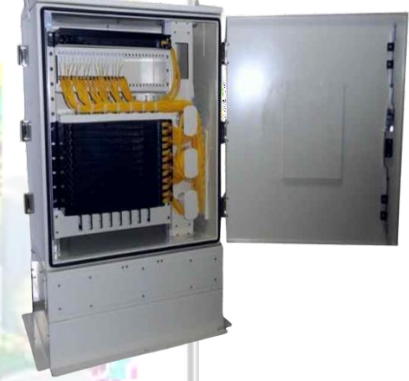
Fiber Distribution Hub
